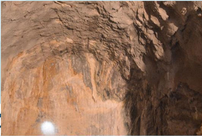
Alteration fractured zone in 2# access tunnel
