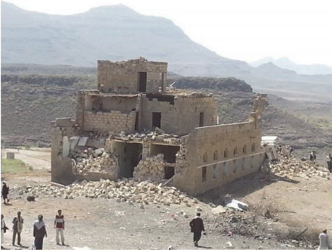
The remnants of the house of Sheikh Muhammad al-Haddi, which was damaged in an airstrike on August 8, 2015. The home had attracted many visitors, as the only house in the village with a generator, and there were about 70 people present at the time of the bombing. Noone in the house was wounded. © 2015 Private
