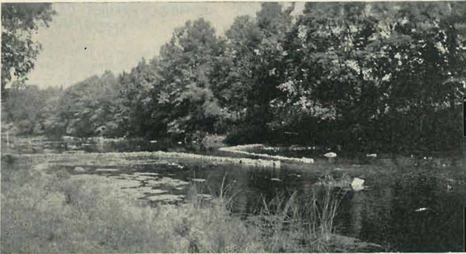
This special V-type deflector, was built with the intention of cutting a channel in a wide shallow of the stream.
