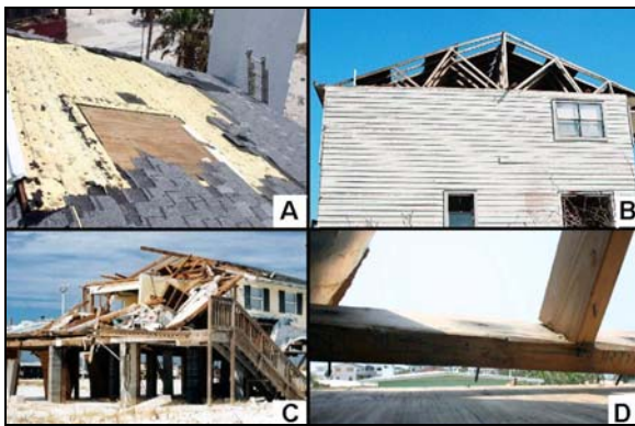
Figure 16. Examples of wind damage to buildings elevated on timber pilings: a) removal of roof covering, b) gable end and roof deck failure, c) windward wall failure, and d) nailed wall bottom plate pulled out of the floor.
