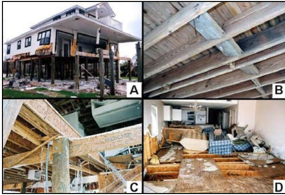
Figure 15. Damage to floor systems from wave action: a) loss of floor girders, b) rotation of blocking, c) stacking of floor joists, and d) uplift of the plywood subfloor.
