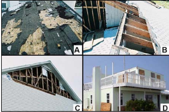
Figure 12. Examples of wind damage to buildings on concrete slab foundations after Hurricane Ivan: a) displaced roof covering, b) uplift of roof decking, c) removal of gable end/siding, and d) complete roof failure.
