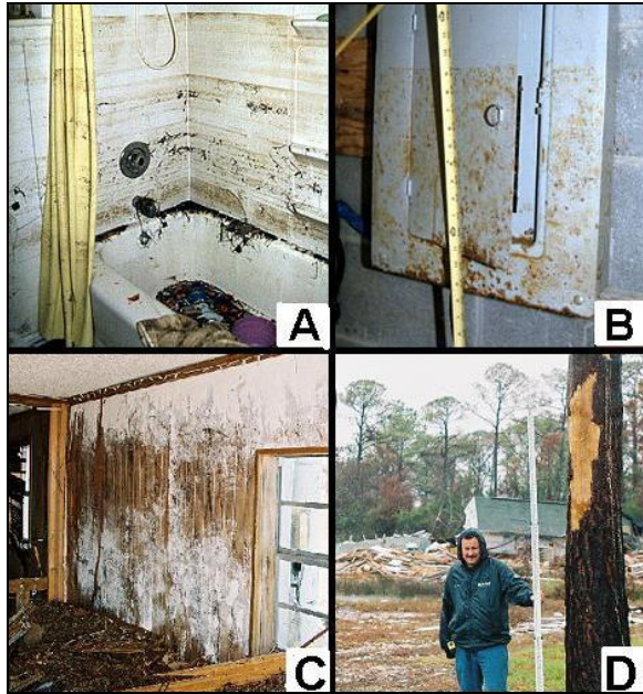
Figure 4. Indications of the height of water: a) dirt line in bathroom, b) rust line on metal fuse box, c) scrape marks on paneling, and d) scrape marks on trees.
