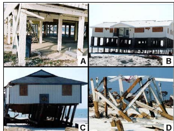
Figure 14. Damage to pilings from wave action: a) breaking of cross bracing, b) erosion of sand around the pilings, c) rotation of pilings, and d) breaking of pilings.
