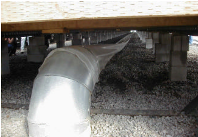
Figure 5. Under-bench heating system.
