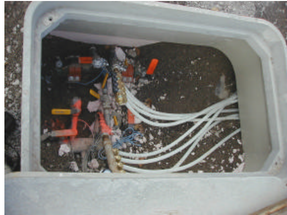
Figure 3. Details of the main control valve box.
