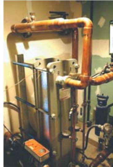
Figure 4. Photograph of the heat exchanger between the City geothermal district heating system and the brewery secondary heating loop.
