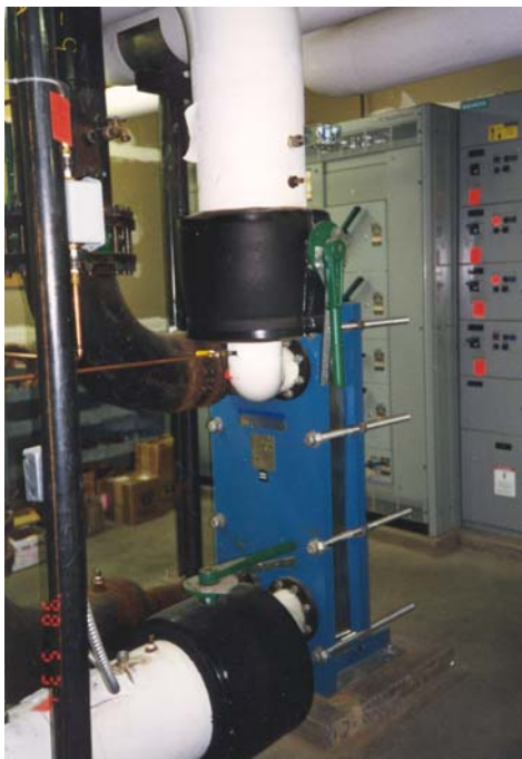
Figure 2. Photograph of one plate and frame heat exchanger at the Inn of the Seventh Mountain.
