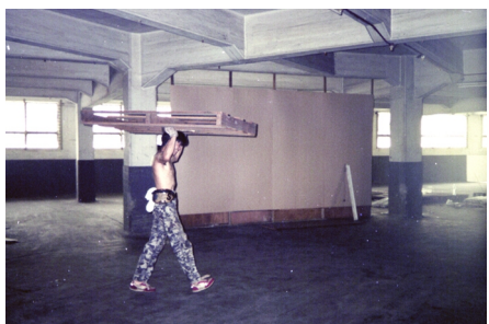
Wooden pallets scattered all over the warehouse in the beginning. Ryuichi gathered the pallets and started his installation
