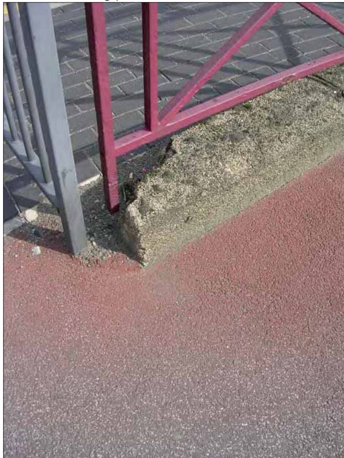
Appleyards Pumping Station railings damage to kerb
