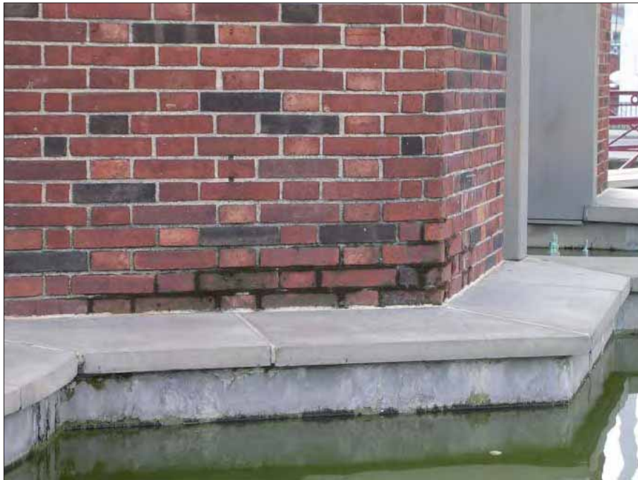
Appleyards Pumping Station evidence of dampness in masonry north side
