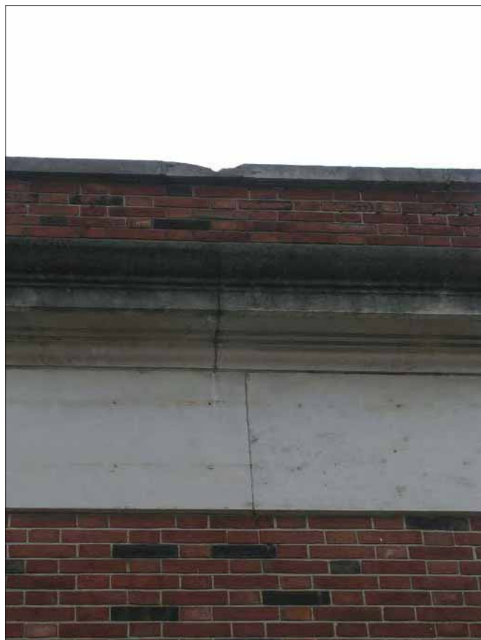
Appleyards Pumping Station minor damage to coping
