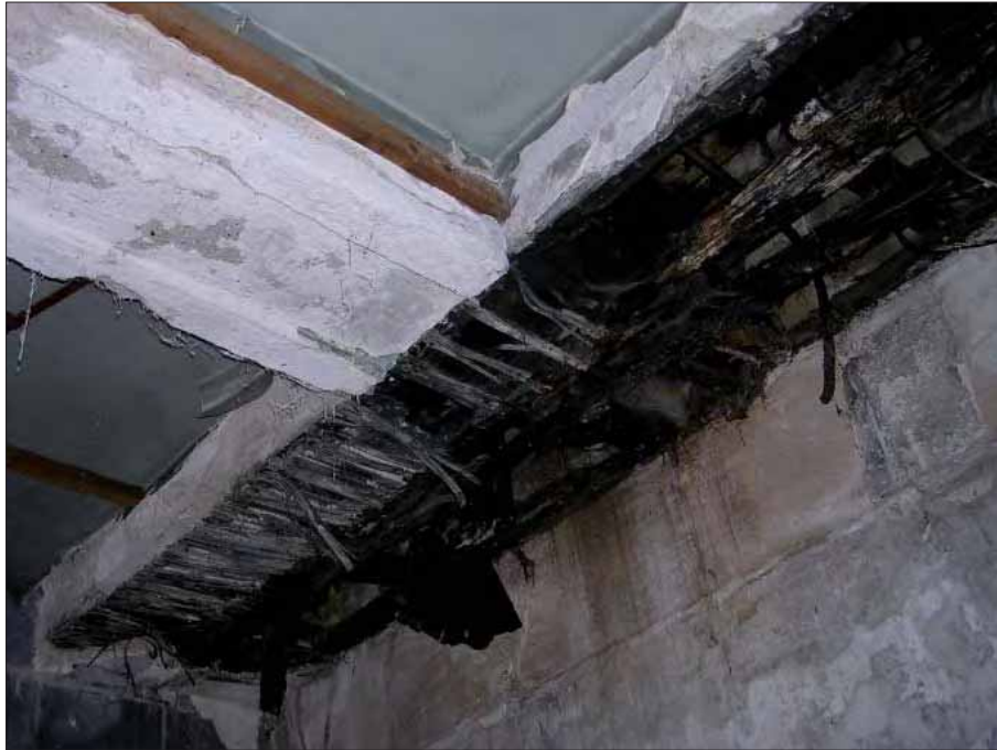
Templar House wet rot on second floor south side
