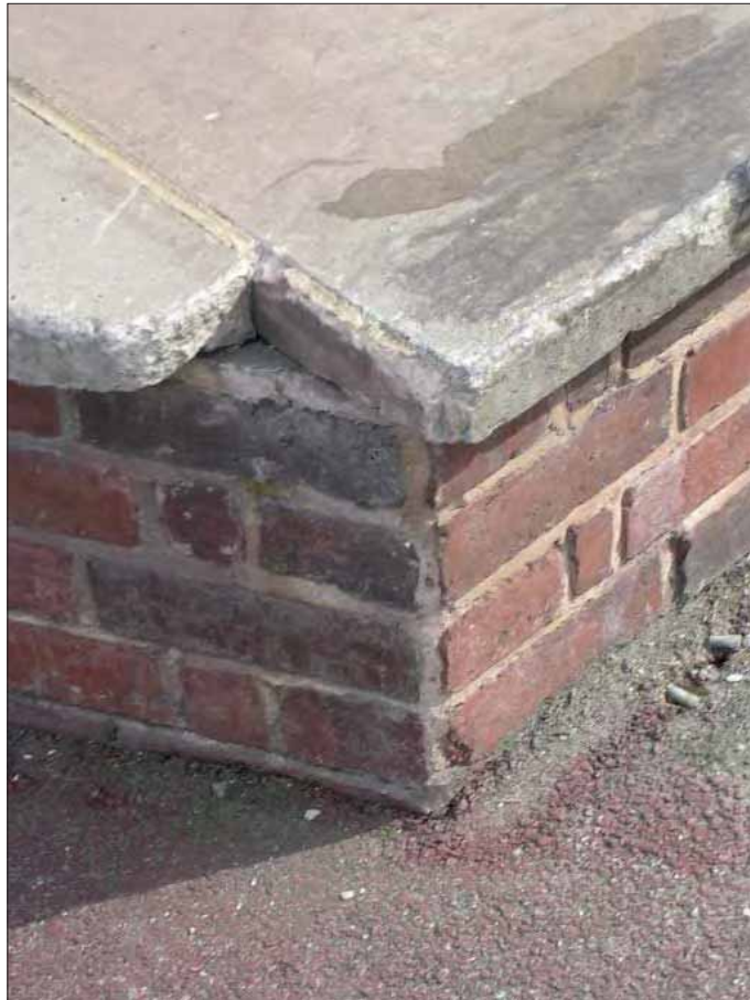
Appleyards Pumping Station damage to modern coping to fountain basins
