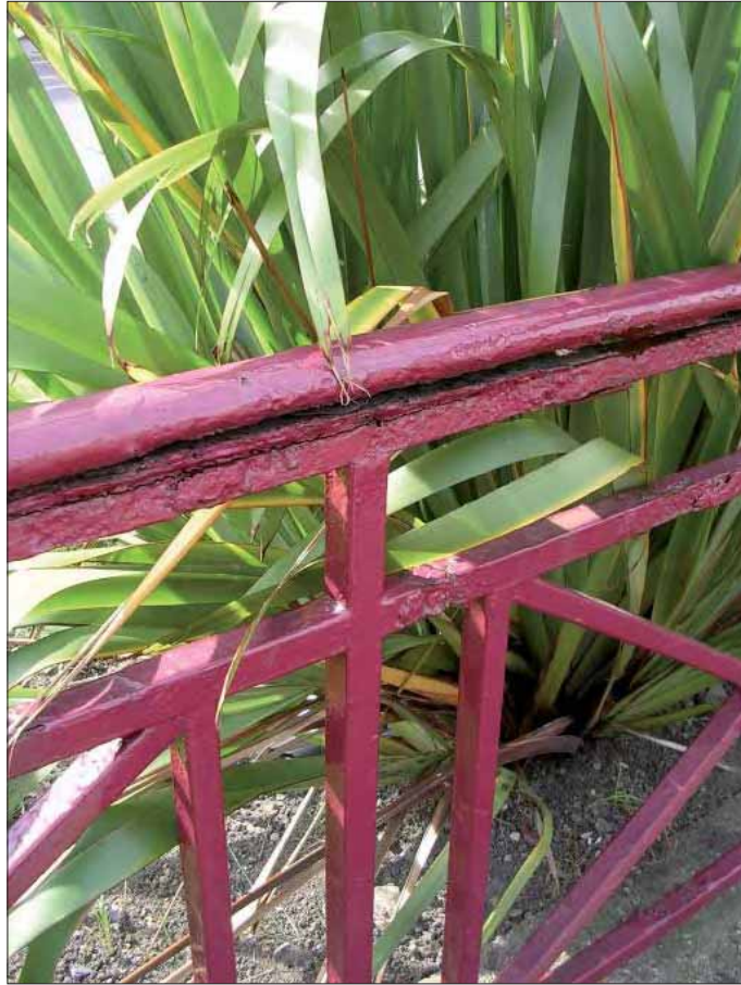
Appleyards Pumping Station railings crevice corrosion
