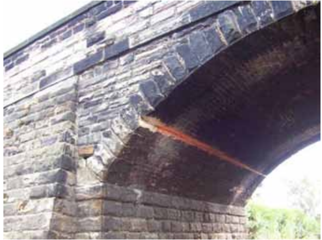
Damage to arched bridge due to a true out-of-gauge load
