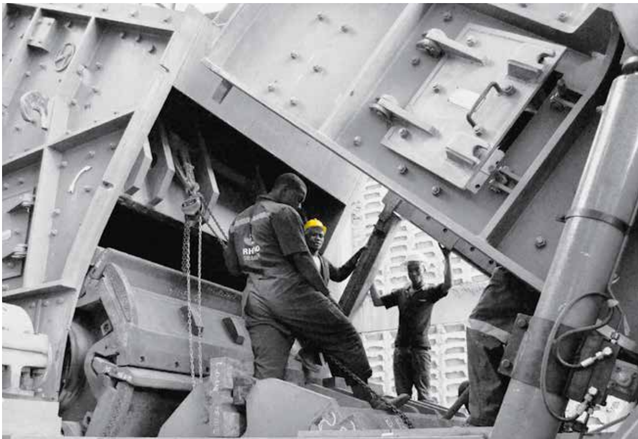
Commissioning of the 800 ton per hour limestone crusher at the Tanga Plant
