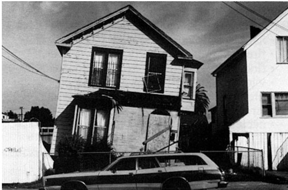
Figure 1. Dwelling in Oakland with Failed Cripple Wall, 1989 Loma Prieta Earthquake
