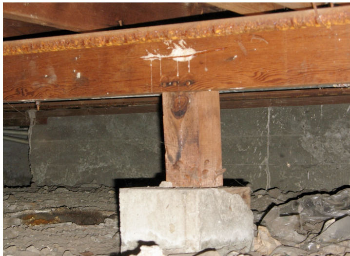
Figure 3. Post Beneath Apartment not Secured to Foundation Pad or Floor Beam
