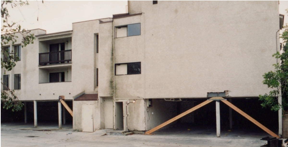
Figure 8. Apartment Building with tuck-under parking in the San Fernando Valley, damaged in the 1994 Northridge Earthquake, temporarily braced to prevent collapse.
