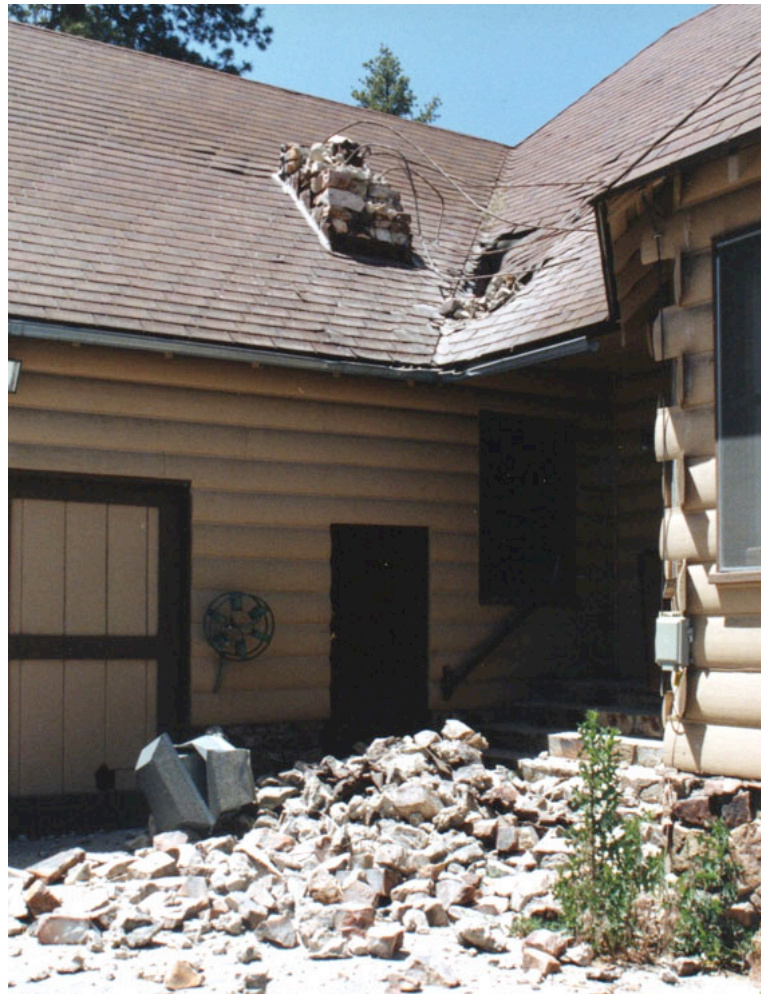
Figure 4. Shattered Chimney – 1992 Big Bear Earthquake
