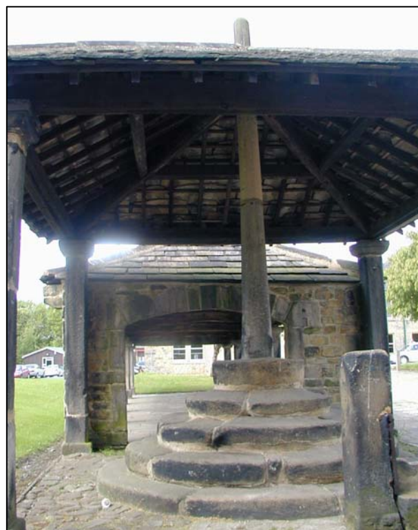
Butter Cross, Stocks and Market Hall (Grade II) – remnants of a bygone age
