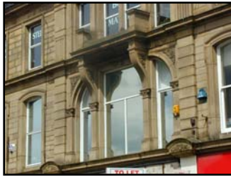
Window detail – 1 st floor Arden House. Typically ornate, reflecting the aspirations of the age.
