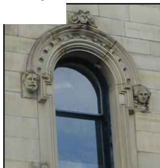
Example of the stone carving detail of some of the more elaborate late nineteenth century buildings
