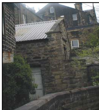
Interesting stone outbuilding with prominent kneelers and recessed openings that nestles to the rear of 1-3 Millgate
