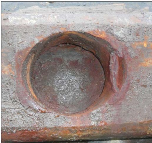
Figure 12: Oval guide hole on retrieved spud pile Source: DMAIB
