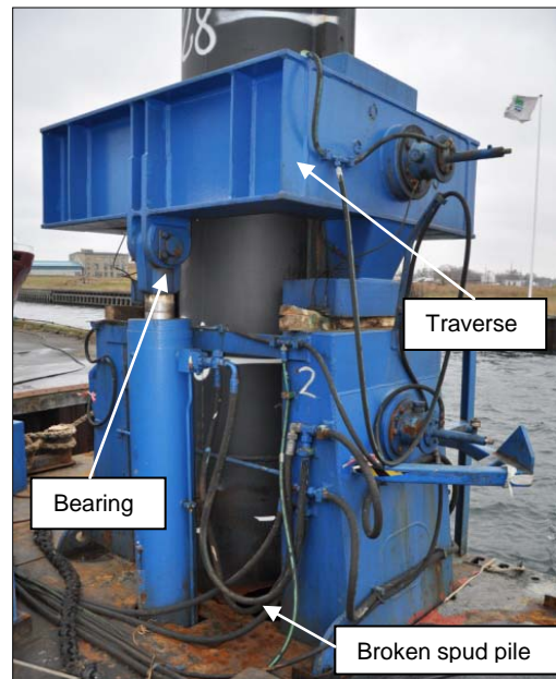
Figure 11: Broken spud pile Source: DMAIB
