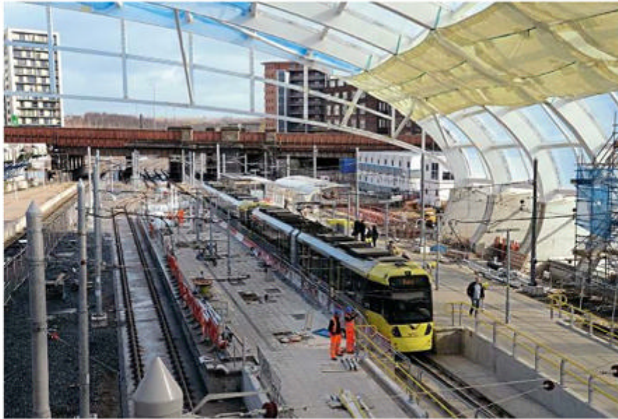
MANCHESTER VICTORIA REOPENS: Metrolink services began using the new stop at Victoria from the end of February, following 11 months of rebuilding work. The track layout has been altered and new platforms built as part of a wider project to refurbish Victoria main line railway station. Trams to Bury and Rochdale started using the stop from February 18, while through services to and from the city centre called from February 21. Further work is needed, but when finished, the stop will have three platform faces instead of the previous two. The state of progress is pictured on March 4 as No. 3017 arrives with a service for Rochdale. Picture: PAUL SENIOR
