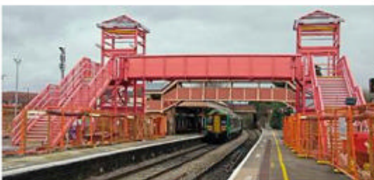
STRATFORD FOOTBRIDGE: The new footbridge at Stratford-upon-Avon seen on February 14 with unit No. 172336 in the station. The lift shafts will have brick infill to give a traditional look. There is a campaign to reopen the line beyond the DMU to Honeybourne as a diversionary route. FRASER PITHIE
