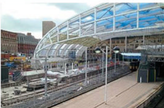
MANCHESTER ROOF: Nearing completion: The new roof structure at Manchester Victoria looking south towards the recently reopened and extended Metrolink tram stop on March 4. MIKE HADDON
