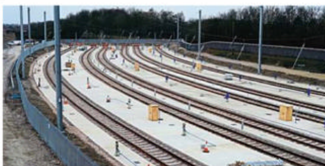
THAMESLINK STABLES BUILT IN PETERBOROUGH: Six new stabling sidings for the new Class 700 Thameslink trains, complete with controlled emission toilet disposal facilities, are nearing completion at Peterborough. The sidings have been built on the site of the old New England steam shed. PAUL BIGLAND
