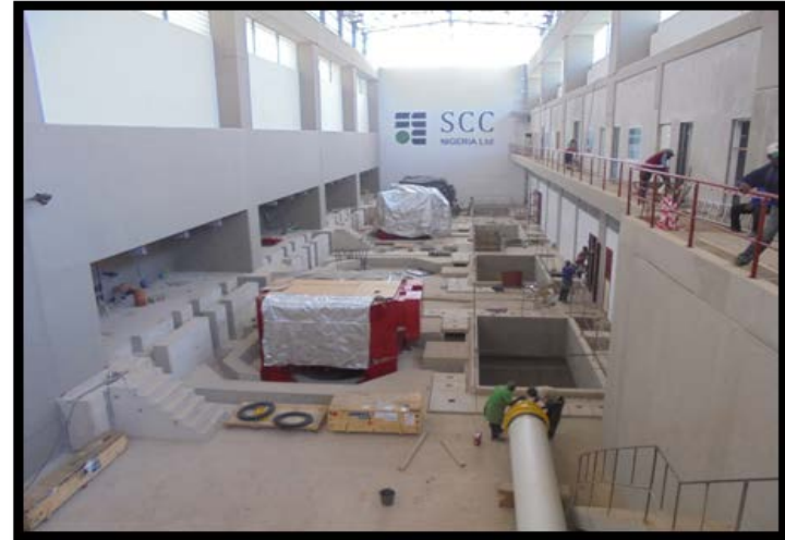
VIEW OF THE GENERATORS IN POSITON
