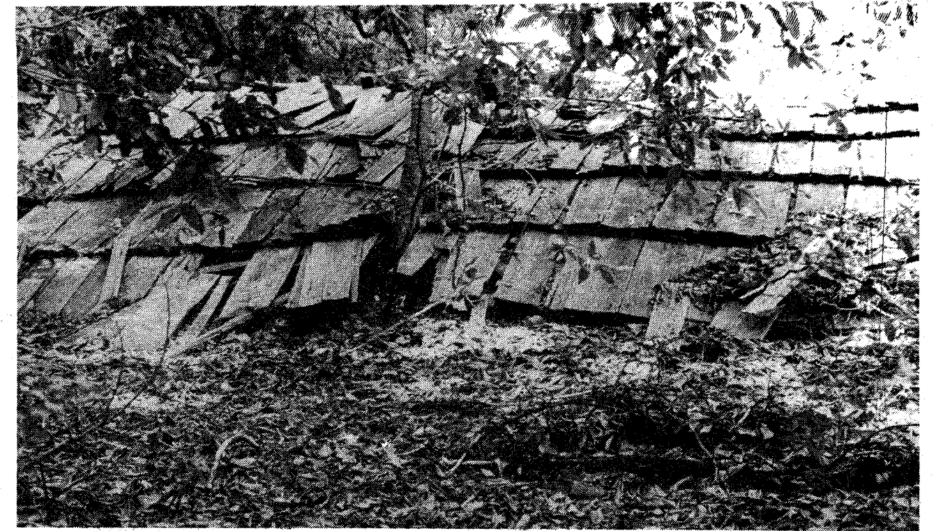
THE ROOF of the Kahofer barn. It lies flat on the ground, the support posts having rotted away.
