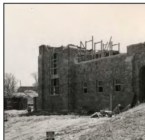
Construction on the Glass Bowl begin in 1936 and was completed a year later.
