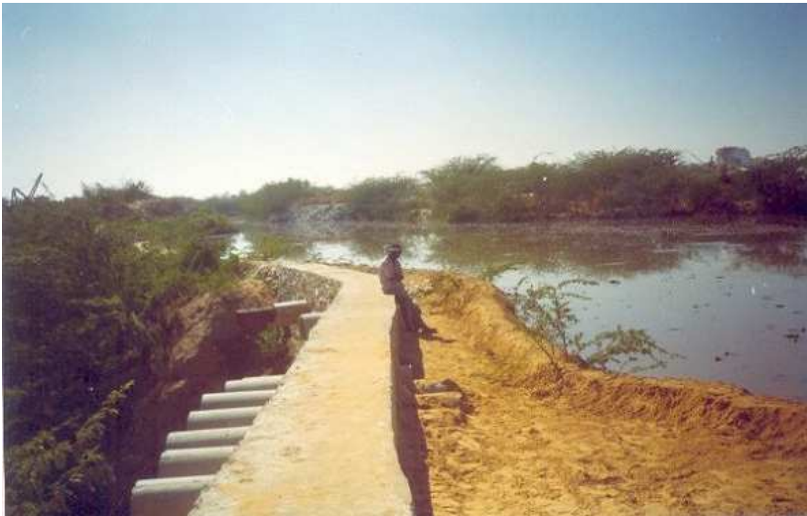
Photo 9: Overflow drains in Kalanada range mines to protect Mosque and school building from flooding leading to ground water pollution, Makrana marble mining area, district Nagaur
