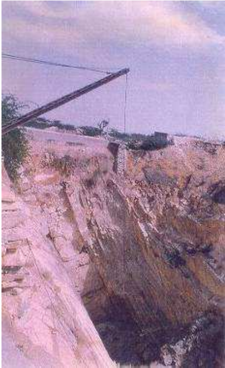
Photo 2a: Undercut in marble band below Gunavati Borawar bypass, Makrana
