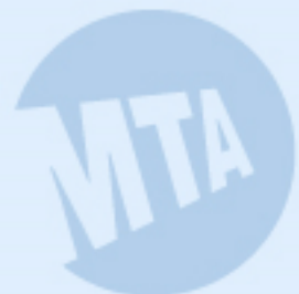
New track wall tiles at lower level platform (on 63 rd Street and Lexington Avenue)
