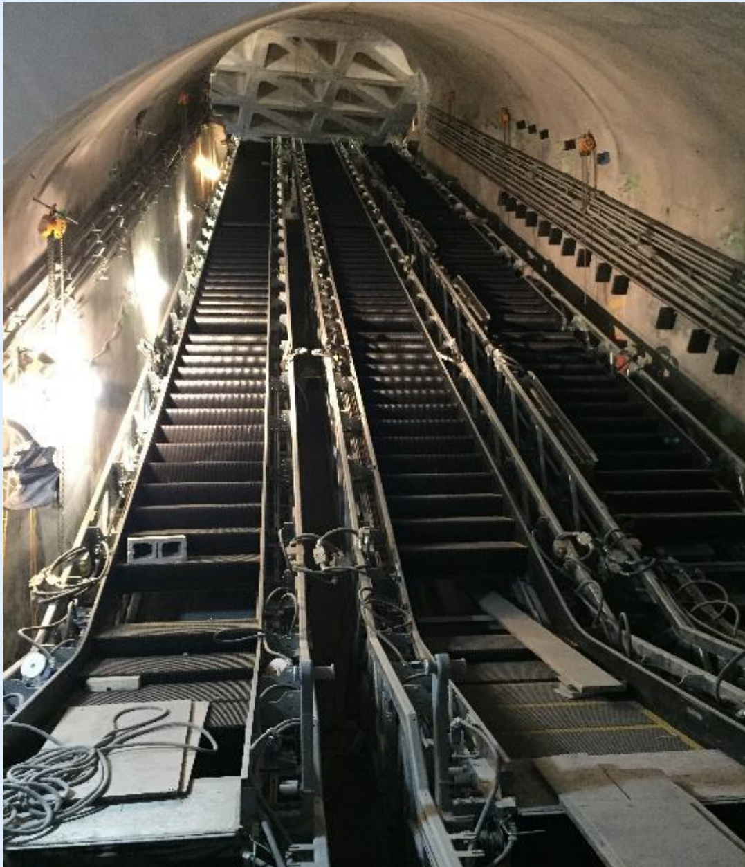
Installation of escalators at entrance 2 (north side of 86 th Street) and architectural ceiling
