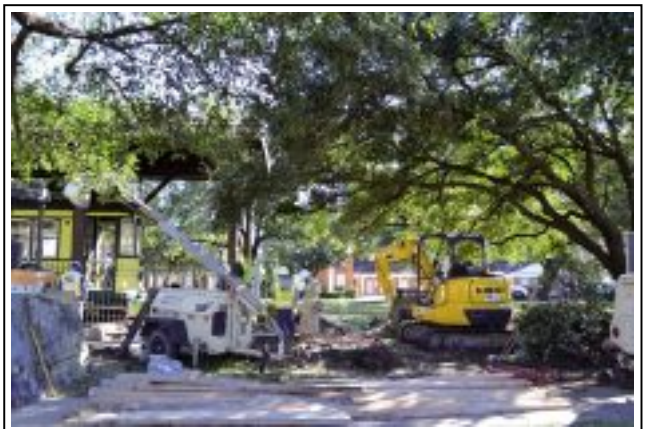
AT&T employees worked round the clock to repair a trunk line severed by construction crews leveling the trolley pavilion. Photo by Michelle Leigh Smith
