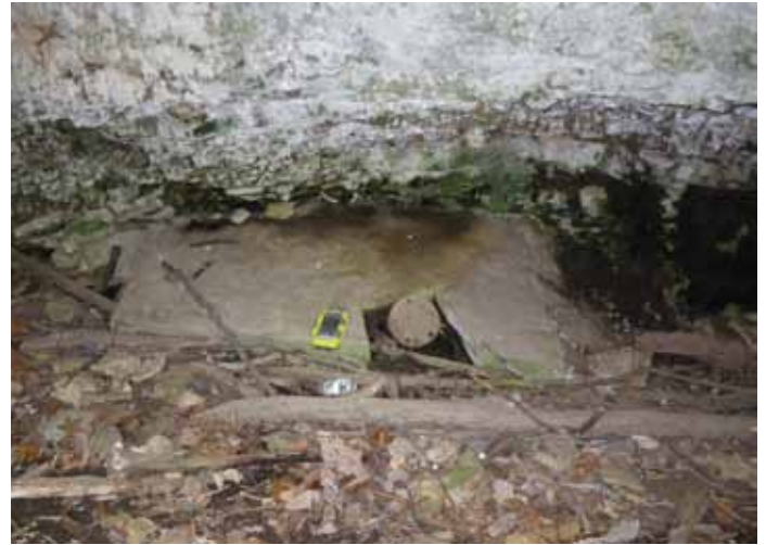
Figure 3: This concrete pad was placed in the largest entrance into Rofkar's Cave I for an unknown purpose. Photo by K. M. Kissell
