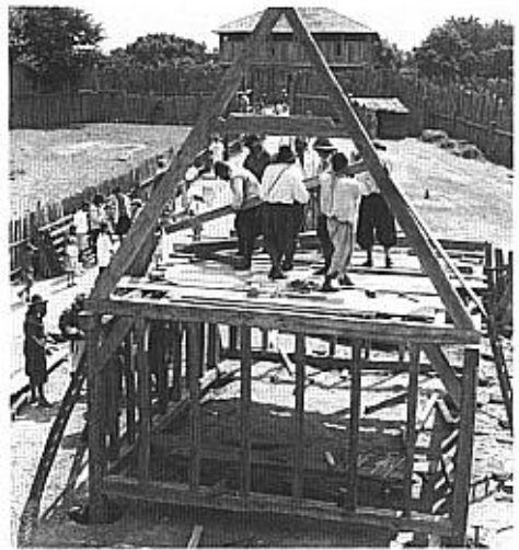
Fig. 14. Standish II under construction, 1993; a section of the older Humphrey palisade is visible at upper left and the new palisade at upper right.
