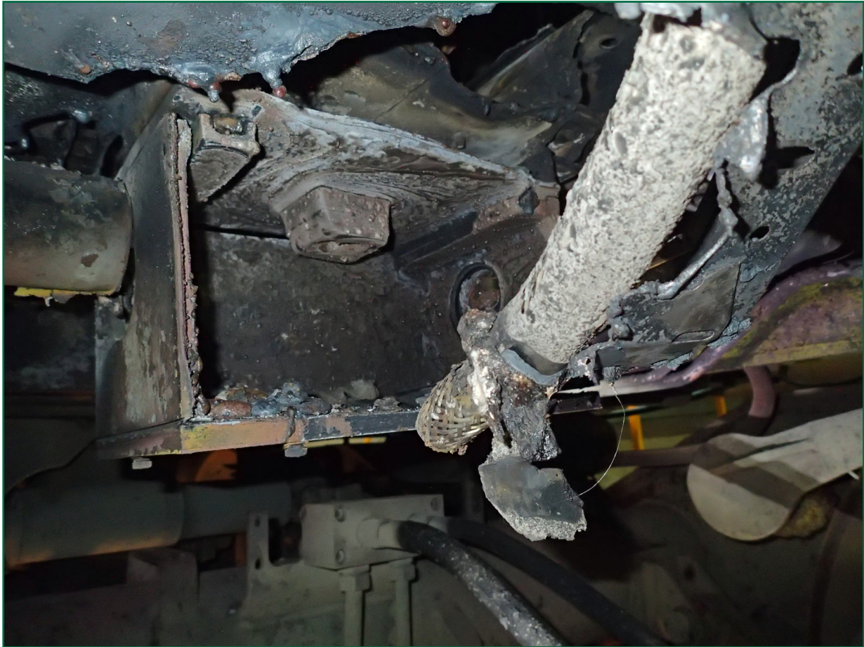
Figure 5: the area where the arcing took place, showing damage to the junction box, cables and structural members
