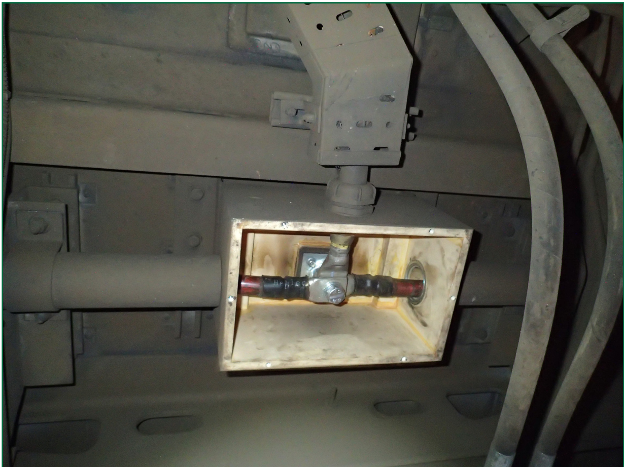
Figure 7: The junction box (undamaged example: lid removed)
