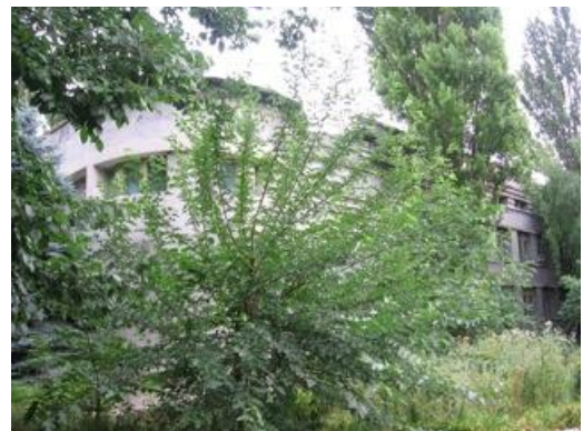
The current state of the film processing pavilion at the Odessa Film Studios, deteriorating and overgrown with weeds.
