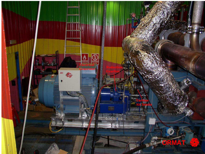
Fig. 2: PCU Commissioning at PSA
