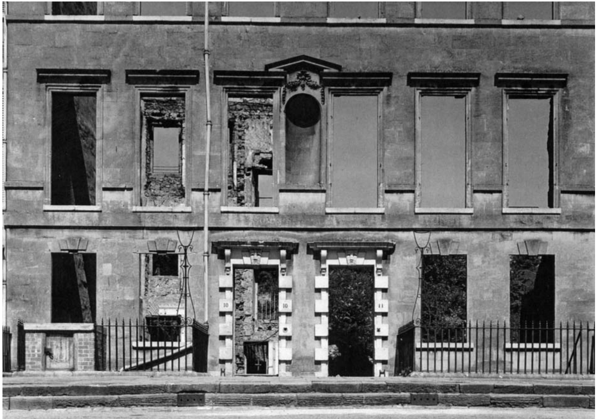
42. Ruined façade of 10-11 Somerset Place 1942 (R F Wills: NMR)
