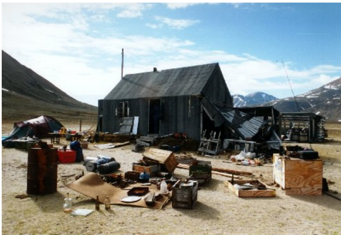
Antarctichavn at arrival. The station was in a poor state. The porch had collapsed. All inventory had to be removed for the renovation to begin.
