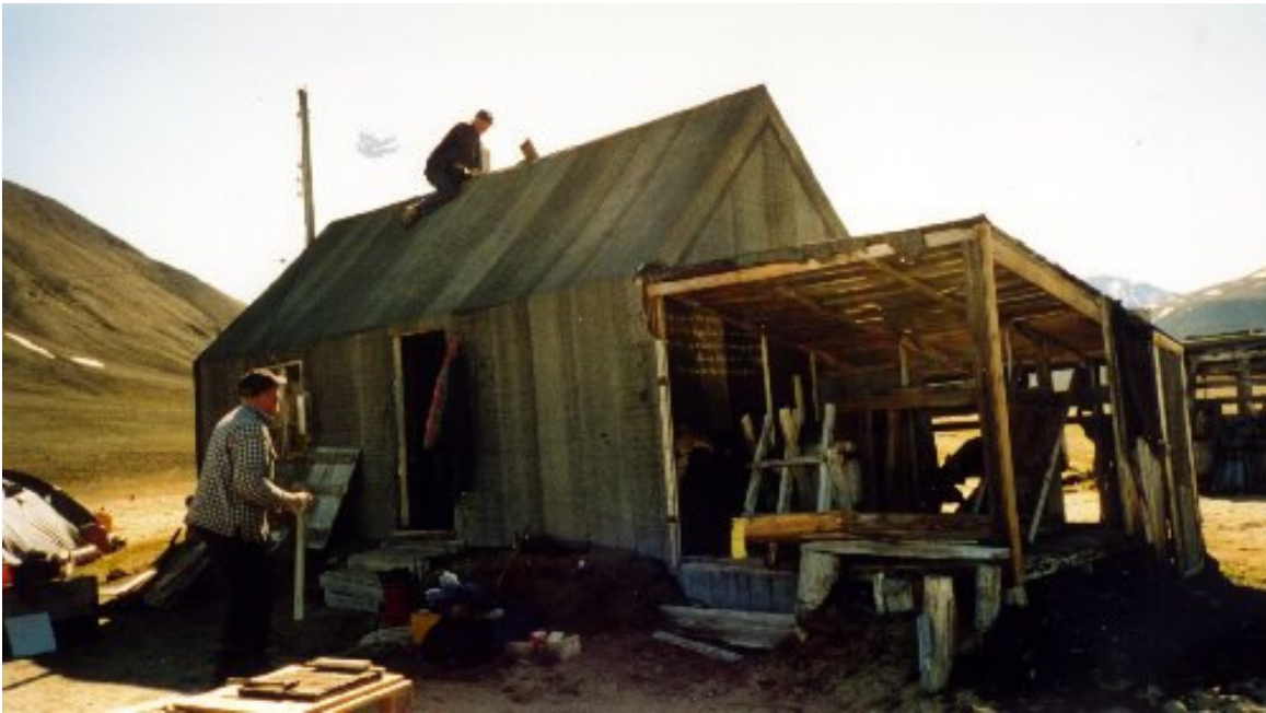
The restoration of Antarctichavn is well under way. The porch has been rebuilt.
