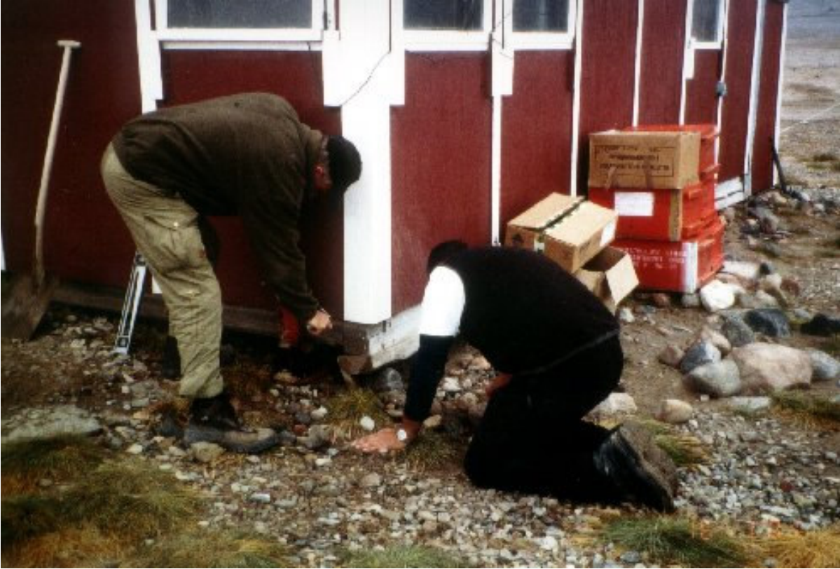
Kap Harald Moltke. The building is levelled.
