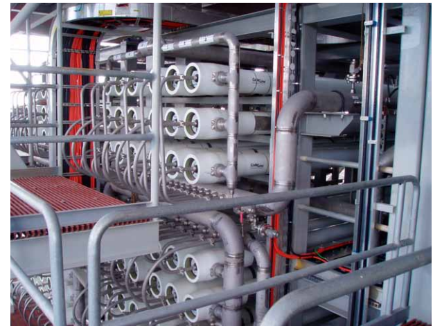
Sulphate Removal Unit Ursa, Gulf of Mexico, USA
