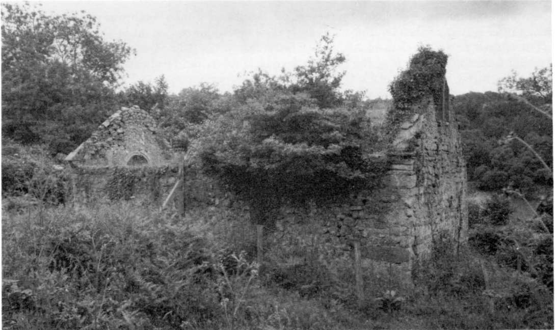
FIG. 9 St James's church; September 1986, before clearance, looking south-east. Photographed by S. Dorey for Gloucestershire County Council.
