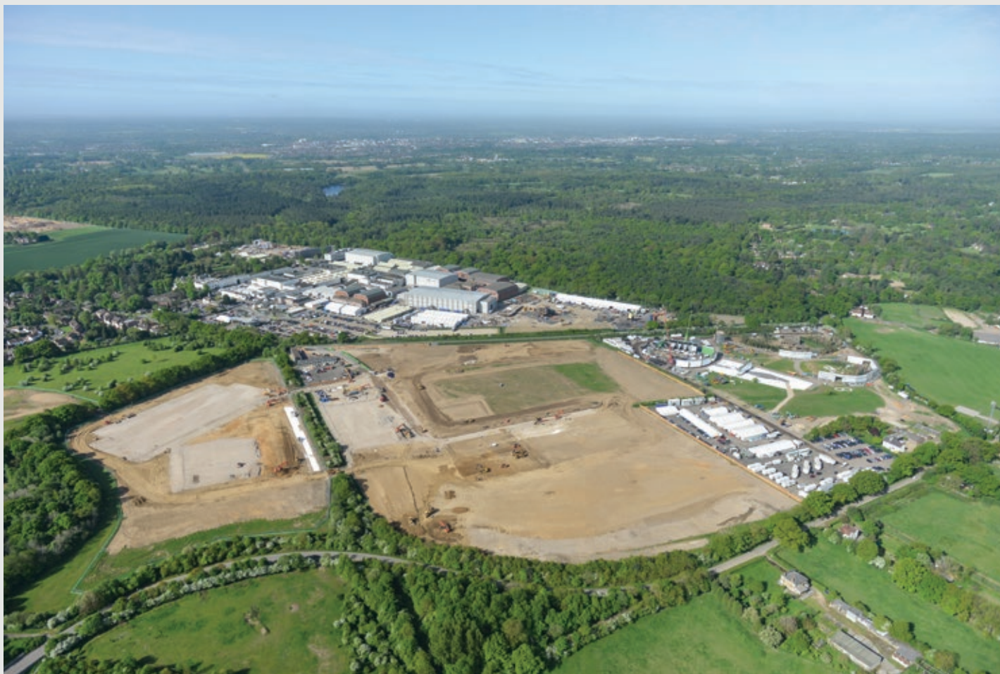
Aerial view of Pinewood Studios showing construction of the Pinewood Studios Development Framework (May 2015) © Pinewood Studios Limited
