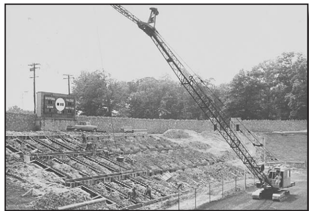
Construction of bleachers in the south end zone in 1966 brought seating capacity to 15,900.
