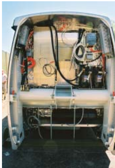
After taking delivery of the Swiss-made train cabins, Schwager Davis, Inc., performed wiring and final assembly of the vehicles on-site.
