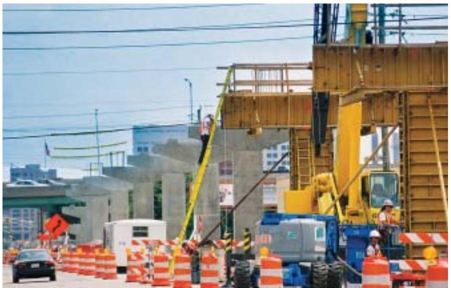
The total scope of work under SDI's design/build contract included all traffic control and traffic control devices required to minimize negative impacts of construction on the city's established traffic-flow patterns.
