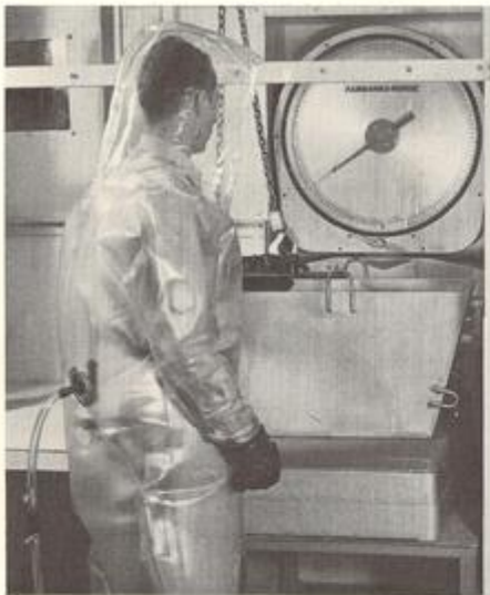
Protective clothing is required in the raw materials handling area of the Fluoride Production Facility (above) to avoid inhalation of the toxic salts. Below, a diagram of the fuel processing system. At right below is the fuel processing containment cell located in the reactor building.
