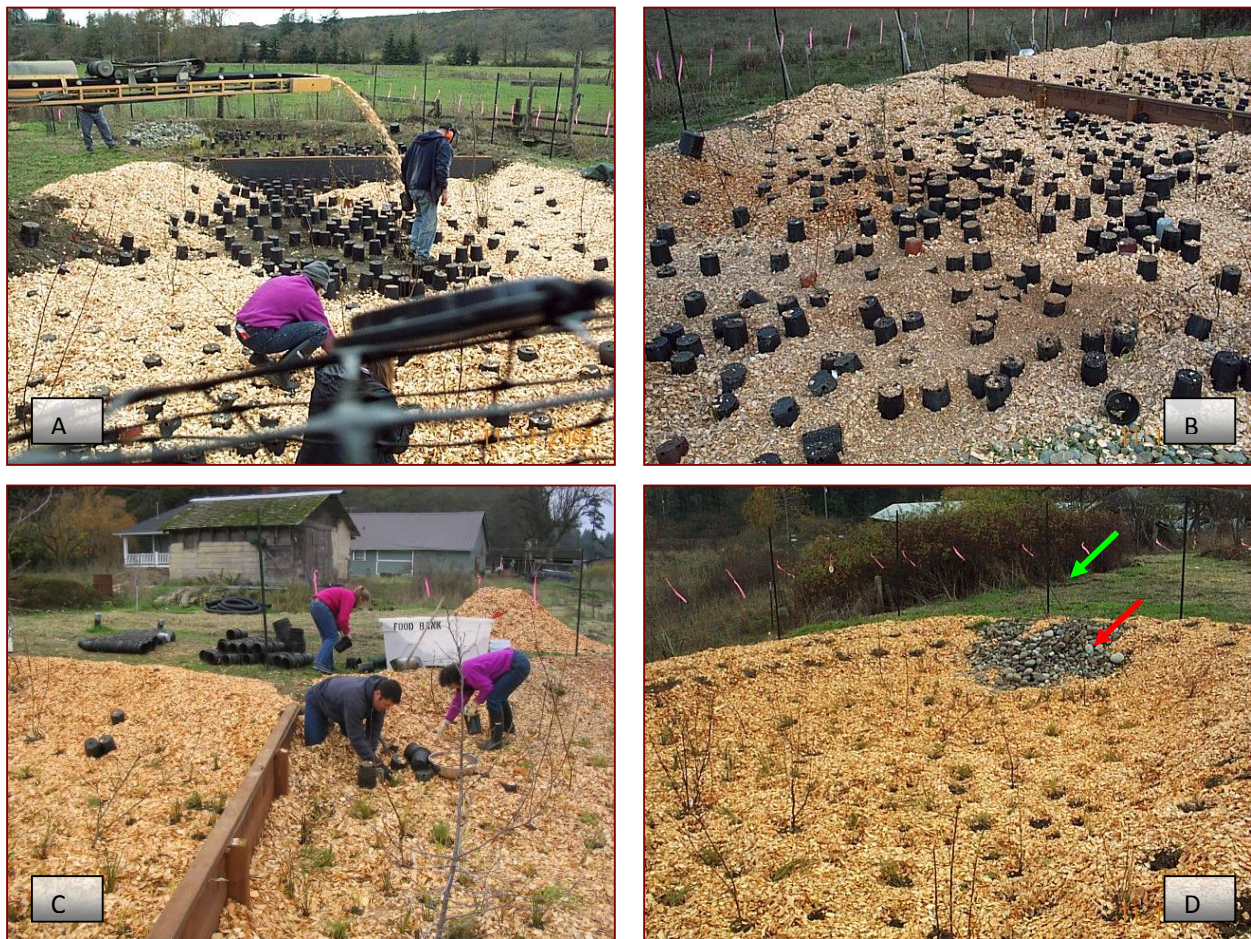
Figure 9. Fungal-Enhanced Mulch was Added by Conveyor System (A), Spread Around the Plants (B), Protective Potting Containers Removed (C), and Energy-Dissipation Rocks Left Uncovered (red arrow) (D). Note deer fence surrounding cells (green arrow).
