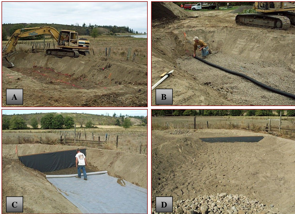
Figure 5. Construction of Twin Biofiltration Cells: (A) Excavation of Twin Cells; (B) Placement of Perforated Underdrain Pipe in Gravel Envelope, (C) Placement of Permeable Landscape Fabric and Impermeable Barrier Between Cells (red arrow), and (D) Energy-Dissipation Rock at Surface Outlet with Layer of Sand and Organic Material
