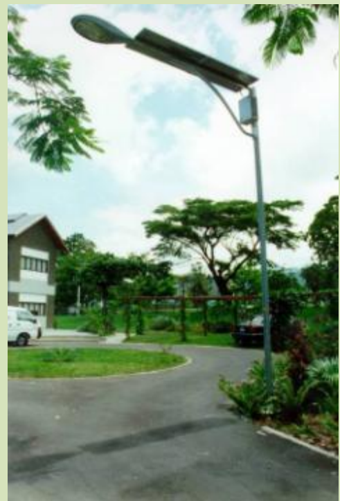
Solar panel on outdoor lighting at Institute of Sustainable Development, UWI
