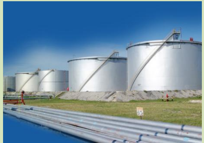
Petrojam Storage Tanks
