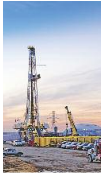
A fracking rig at the Barnett Shale in North Central Texas, where Mitchell first began poking for natural gas in the early 1980s.
