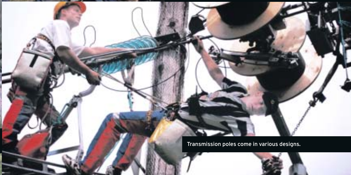
The grid is large and the maintenance demanding.
