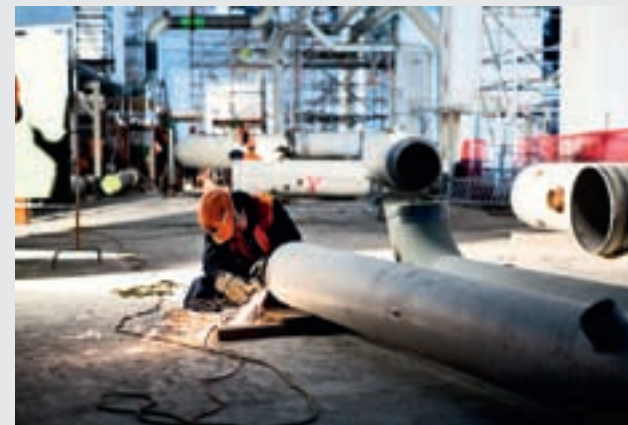
Pipe work at the Moorburg CHP plant in Hamburg, Germany.
