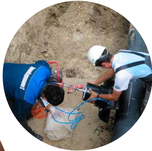
Despite a challenging environment in Russia, Aliaxis completed several major projects including the supply of a safe, efficient and user-friendly pipe system for the water supply of a prestigious apartment complex in the Seven Winds district in Volgograd.
