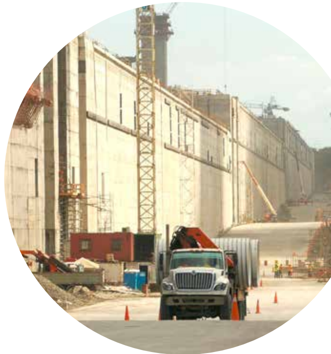
Based on the group's expert technical assistance and ability to deliver and support major projects at short notice, Grupo Unidos Por el Canal (GUPEC) chose Aliaxis for the supply of solid, corrugated and reinforced pipe for the prestigious expansion of the Panama Canal.
