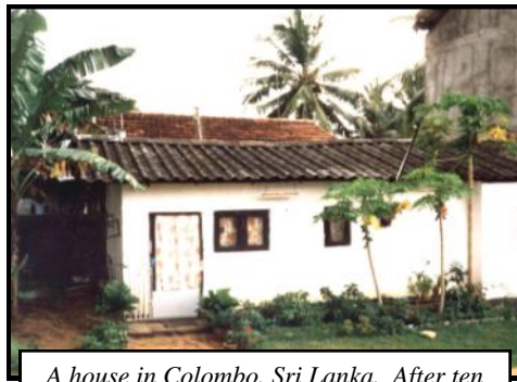
A house in Colombo, Sri Lanka. After ten years the Parry roof is darkened by tropical lichen but is still strong and weatherproof
