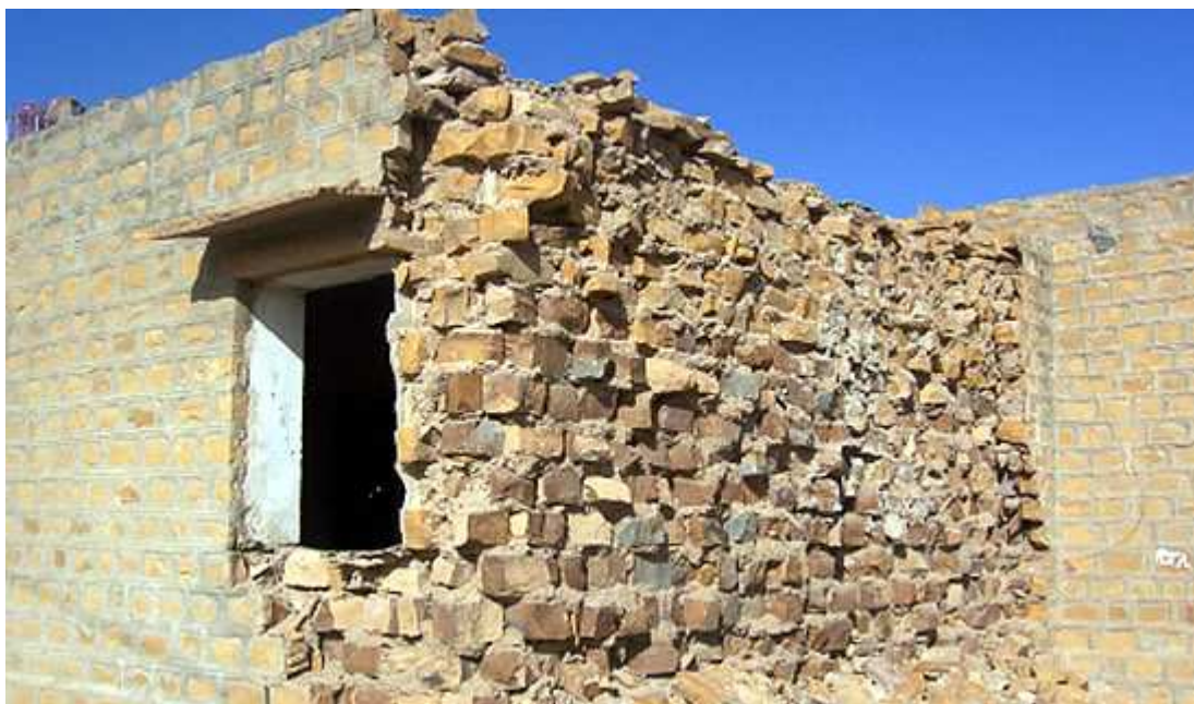
Figure 4: Partial collapse of wall of a school building in Mokhal
