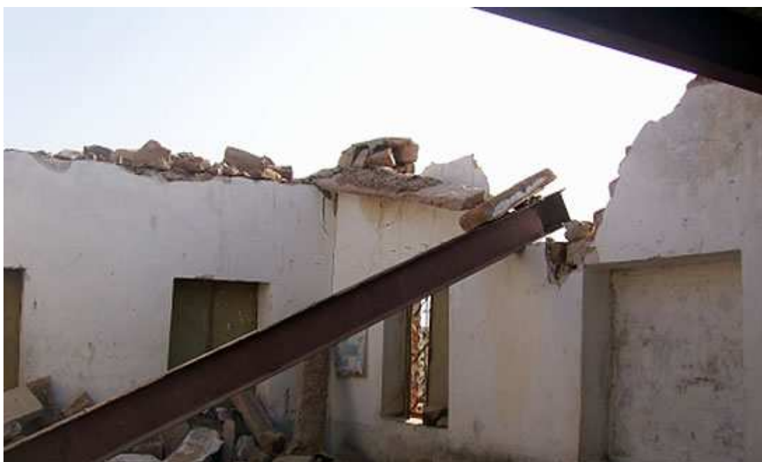
Figure 3: Failure of load bearing E-W wall of Anganbari building in Kurchi village
