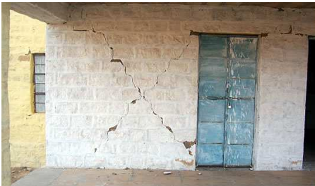
Figure 2: Conjugate joint in wall of School building in Chandan-ki-Dhani
