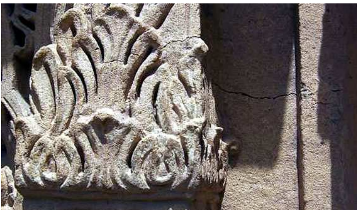
Figure 7: Horizontal cracks developed in pillar of Jain temple Amar Sagar, Jaisalmer
