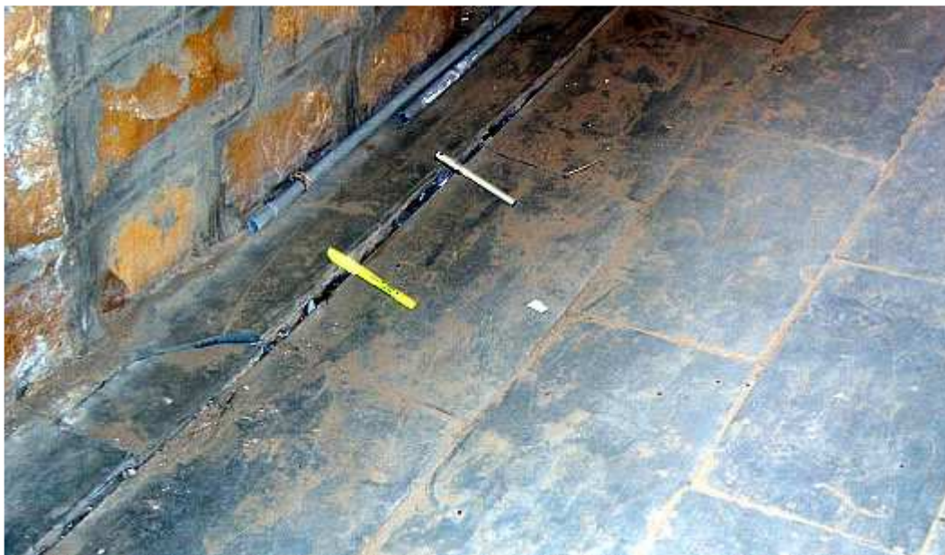
Figure 6: Subsidence in the floor of Kishnai Devi Mangi Ram Girls Higher Secondary School
