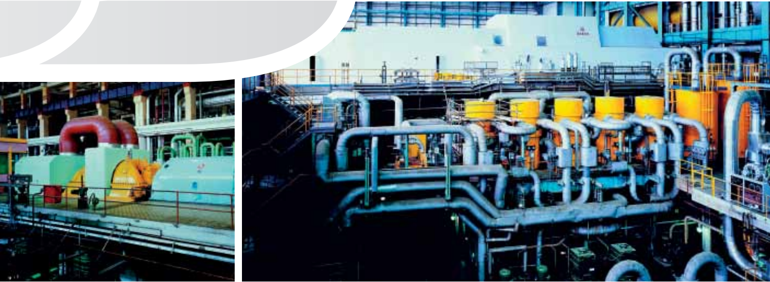
CEZ GROUP - Tisová power plant and coal-fired power plant in Tušimice, Czech Republic
