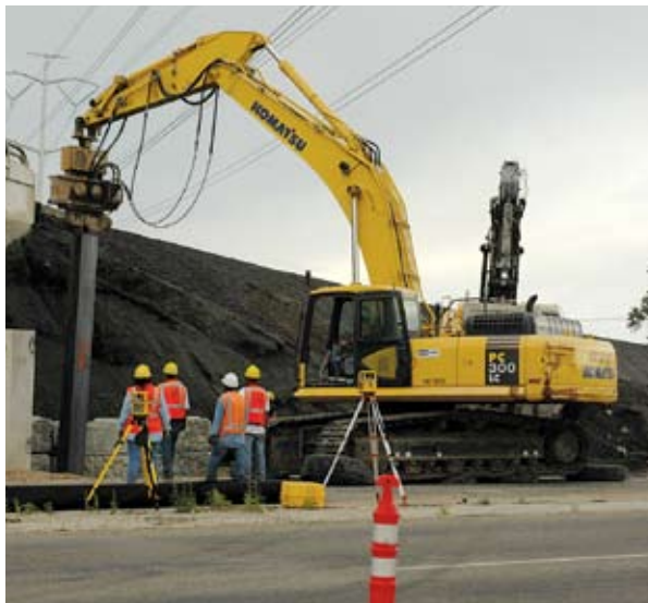
Most Wanted Drilling’s fleet of equipment includes this Komatsu PC300LC-7 excavator. Here, a Most Wanted Drilling operator uses an APE 50 vibratory hammer attachment to push steel I-beams into the ground for a new light-rail bridge connecting Salt Lake City to the Kennecott area.
