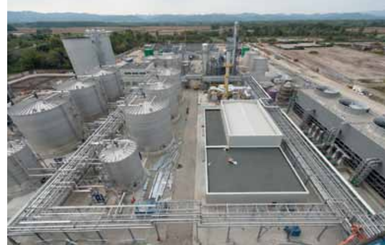
BETA RENEWABLES COMMERCIAL FACILITY
