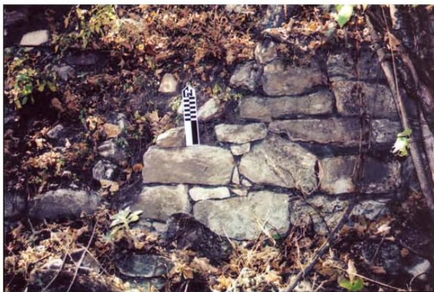
North Retaining Wall (Façade Partially Intact)
