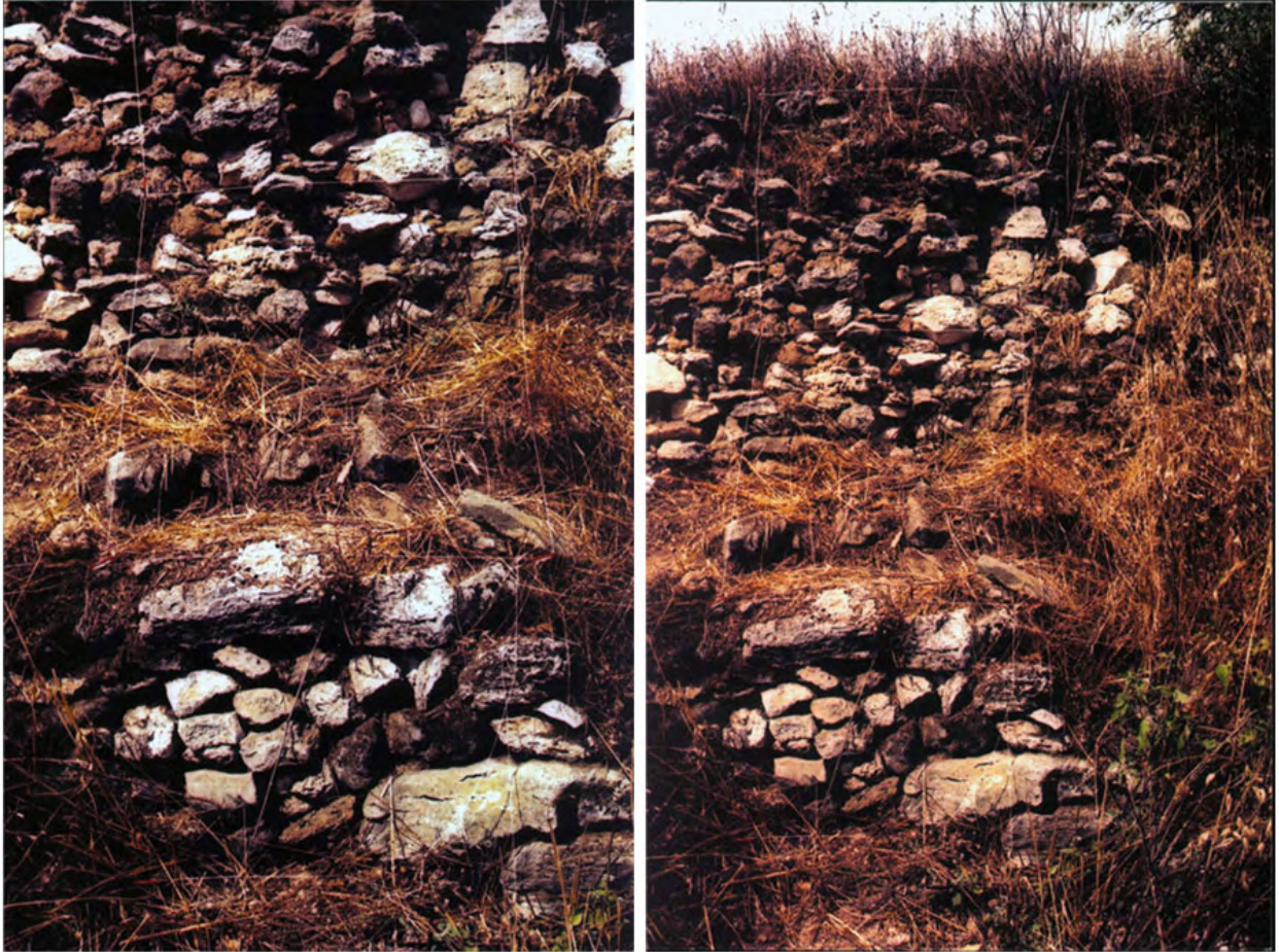
Figure 15. Plaza 1 South Retaining Wall (Rubble Core Exposed).
