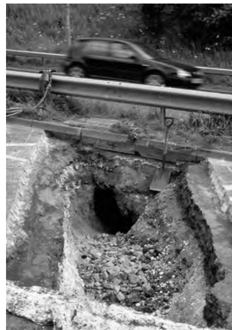
Figure 3. Open void exposed in original fissure, beneath surface of A690 road, June 2003.
