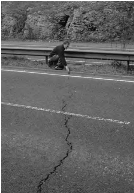
Figure 1. Cracking in surface of A690 road, Houghton Cut, Houghton-le-Spring, City of Sunderland. April 2000.
