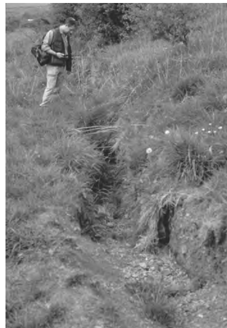
Figure 2. New surface fissure. Hillside west of Houghton Cut 2001.
