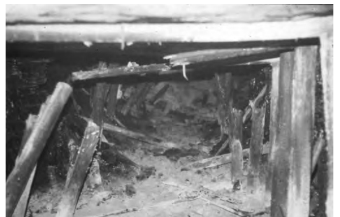
Figure 3. An old open 'bord' in the High Main Seam, Morrison North Pit, Co Durham. (Photo: Andy Witcomb).
