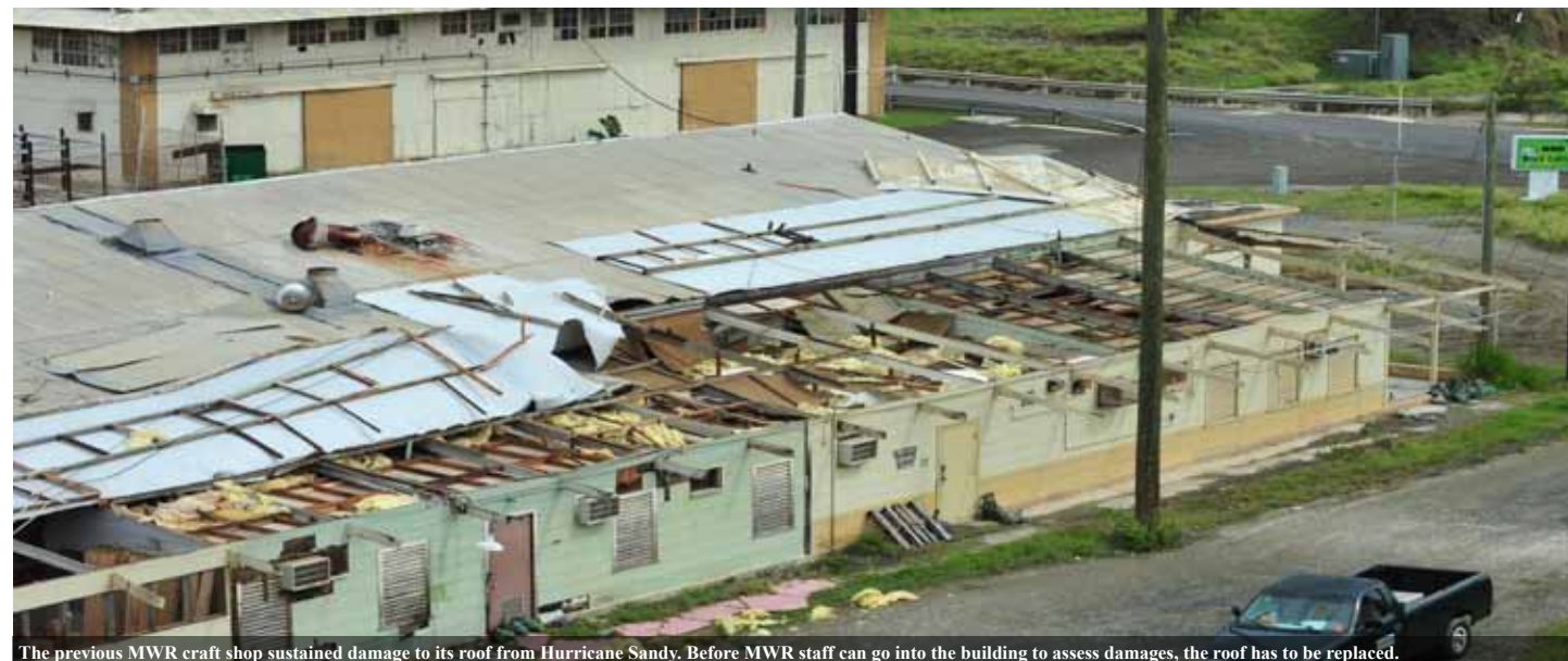
The previous MWR craft shop sustained damage to its roof from Hurricane Sandy. Before MWR staff can go into the building to assess damages, the roof has to be replaced.
