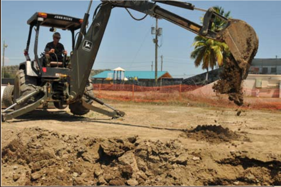
Navy Equipment Operator 1 st Class Christopher J. Grammer, with Naval Mobile Construction Battalion 25, digs a foundation for the future home of a K-Span, March 23. – JTF Guantanamo photo by Army Spc. Cody Black
