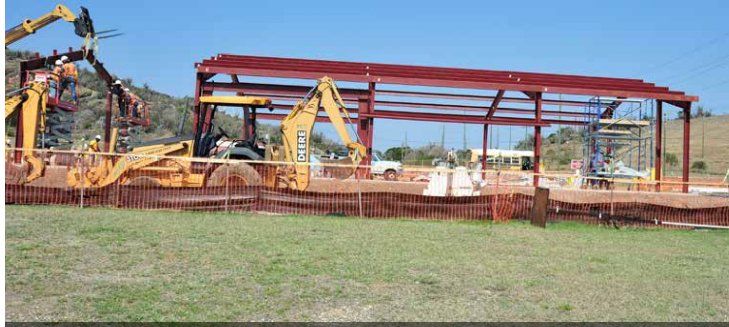
Contractors work on the construction of the new Trooper Chapel, near the Camp Bulkeley Gym recently. The project began in early January to replace the current building, across from the Camp America Post Office, that has sustained weather and mold damage. (Photo by Army Staff Sgt. Michael Davis Jr.)
