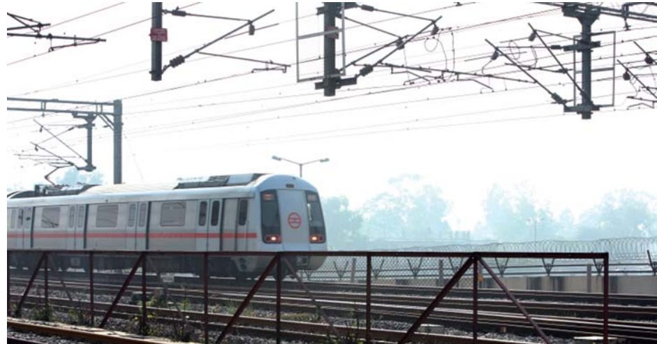
Overhead power supply is a critical element of electric traction systems.
