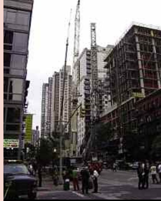
HOMICIDE CHARGE: A New York court has charged crane owner James Lomma and his New York Crane and Equipment Corporation with criminally negligent homicide, assault and manslaughter as a result of a tower crane collapse in Manhattan (above) in May 2008 that killed two workers. The court hearing in March set Lomma's bail at $100,000.
