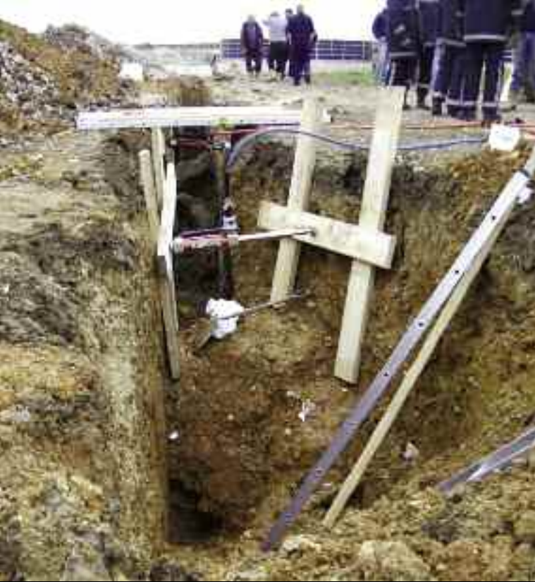
TRENCH HORROR: A Cambridgeshire groundwork contractor was fined £3,500 plus £2,000 costs at Cambridge Magistrates Court in March after a worker was buried alive in this excavation collapse. The Health and Safety Executive prosecuted Anthony John Melvyn Hill, 58, of Sawston, for breaching the Health and Safety at Work Act 1974 and the Construction (Design and Management) Regulations 2007. The accident took place in October 2007 at Penny Farm, near Brinkley in East Cambridgeshire. While one of Hill's employees was in the trench, the sides collapsed, burying him completely. He was rescued by other workers and the Suffolk emergency services. Luckily, he suffered only a broken leg and bruising.
